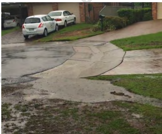
Plate C5.5 – (Photo taken at 10:00 hours) Concentrated flow discharging from gutter in Linden Crescent, Cranebrook.
