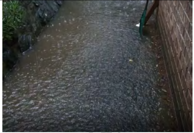
Plate C1.2 – (Photo taken at 19:00 hours) Floodwater ponding at side of property that is located on Soling Crescent, Cranebrook.
