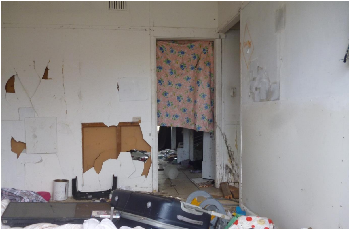
Figure 14: Internal view of living area in Duration Cottage located at 45 Carinya Avenue.
