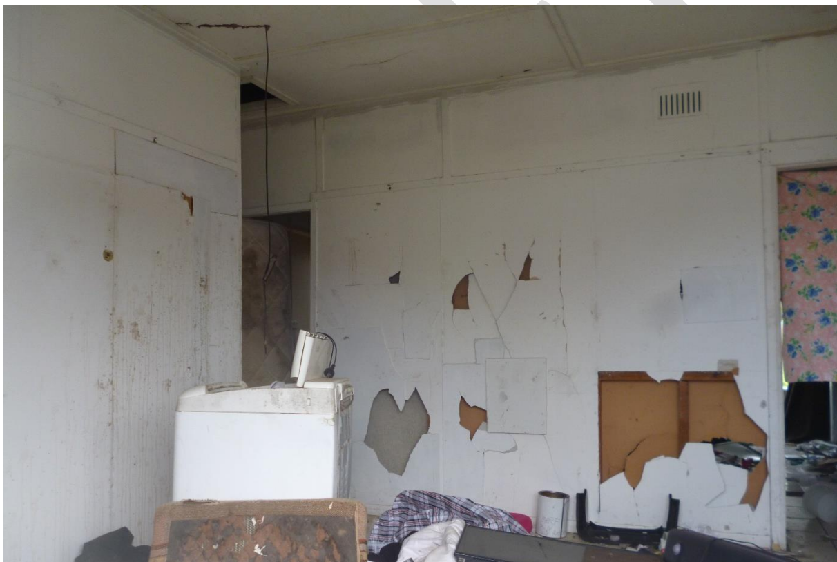
Figure 13: Internal view of living area in Duration Cottage located at 45 Carinya Avenue.
