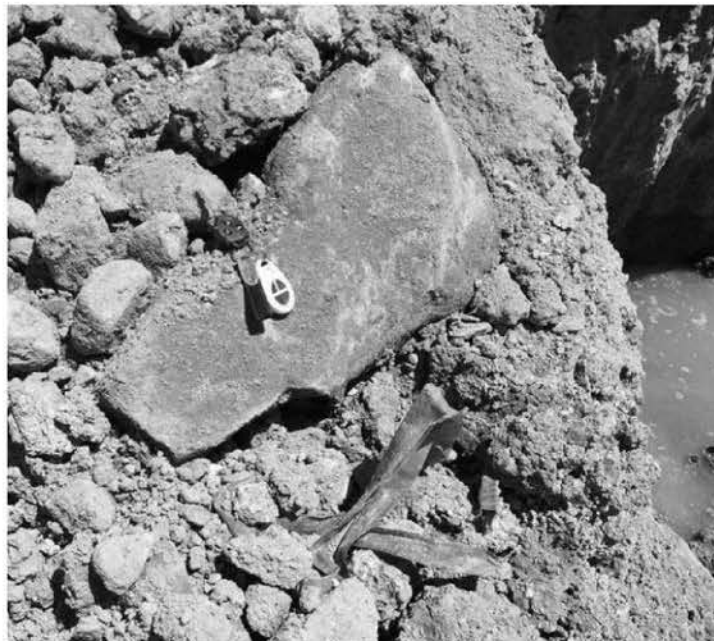
Photograph 14 – Photograph taken from within the excavation for the Armoury Road remedial works located north-east of the Armoury Road / Navy Road roundabout within Stage 1 of JSE. View of the state of the fill material including sandstone boulders and plastic within the fill
