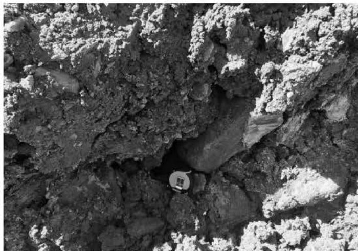
Photograph 9 – Photograph taken from within the excavation for the Armoury Road remedial works located north-east of the Armoury Road / Navy Road roundabout within Stage 1 of JSE. View of the state of the fill material including possible voids and sandstone boulders within the fill
